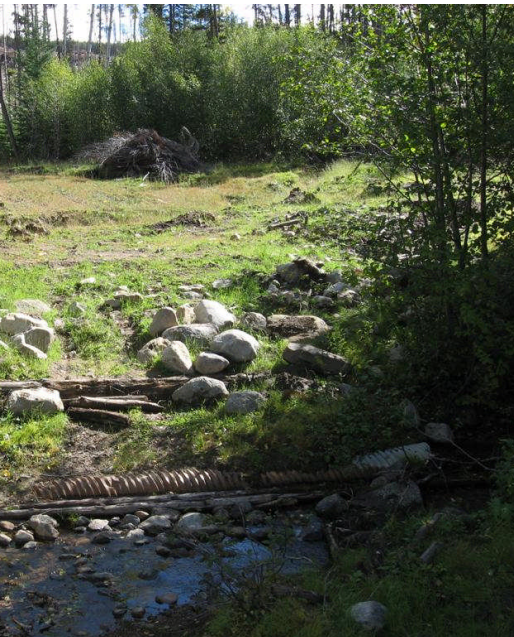
Rehabilitation of a fish stream crossing; note the grass seeding to minimize sediment input to the stream. The inset picture is a view taken during the 2009 audit when the crossing was still active.
